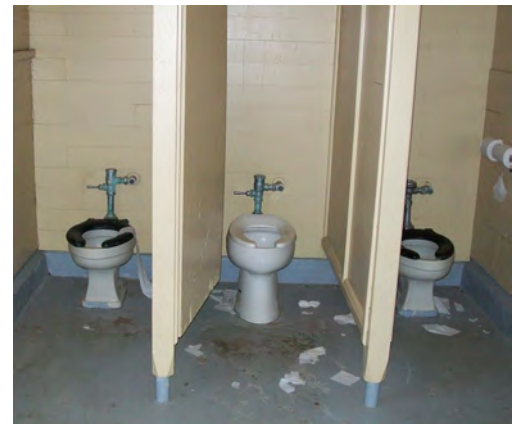
Below- Field House facilities in need of repair.
